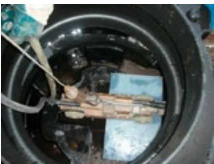
Inspection of flushing results with pan and tilt camera, camera on the maintenance console in the start shaft of a SediPipe L system
