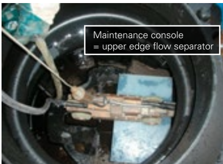
Inspection of flushing results with pan and tilt camera, camera on the maintenance console in the start shaft of a SediPipe basic system
